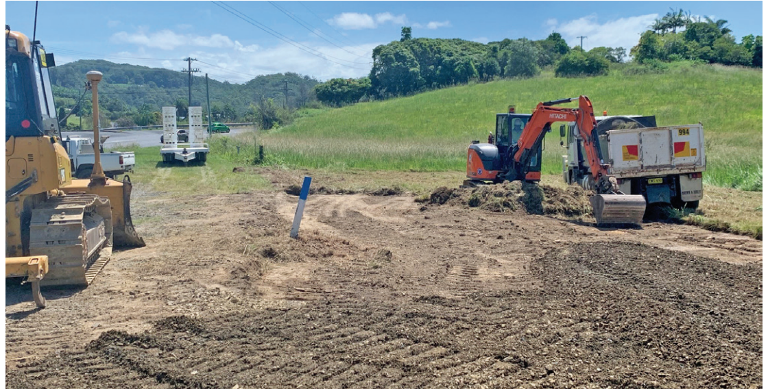
WORK UNDERWAY: Work is underway on the Coffs Harbour bypass at Coramba Road thanks to $1.4 billion investment by the Federal Government.
